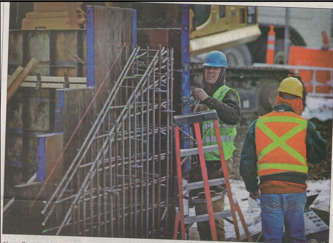
Above: Terry Sinnema, of Belgrade, left, a subcontractor working for Anderson Precast, stops to talk with Caleb Minnick, a civil engineer with CTA Architects and Engineers, while working on forms for a retaining wall on the Main Street/View Vista Drive over Fleshman Creek, Friday. Below: Craig Kamps, of Livingston, who is a land surveyor with CTA, stakes out the area for new storm drains on View Vista Drive over Fleshman Creek, Friday.
