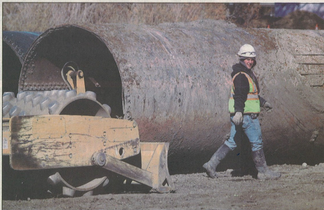
Damian Harris, with Sime Construction walks past a section of a culvert made from a railroad tank car that was dug up on H Street as part of the ongoing Fleshman Creek restoration project, Wednesday.
