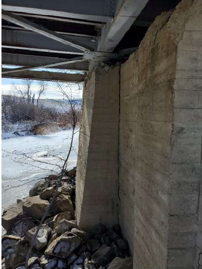
Figure 7: Crack in west retaining wall
