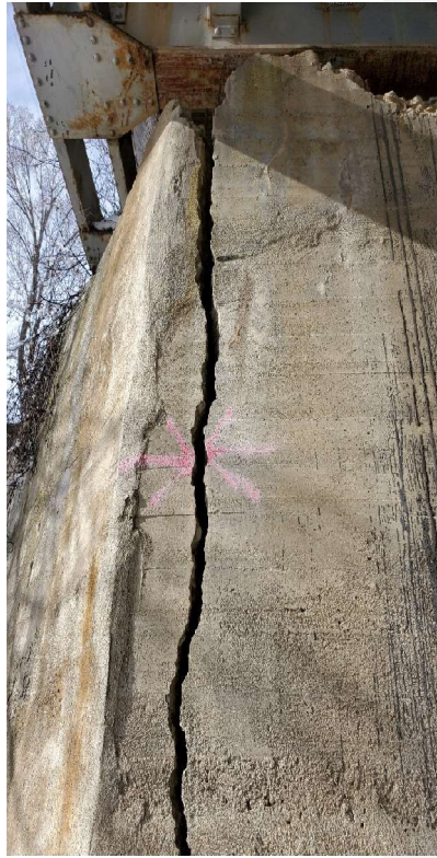
Figure 5: Large Crack in retaining wall
