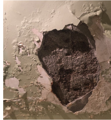
Water damage in the third floor former secretary's office (left).
