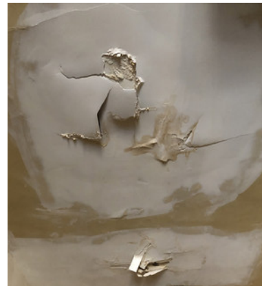
Damaged ceiling in the third floor hallway.
