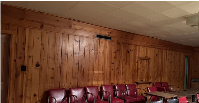
Wood paneling and tiled ceiling in one of the third floor rooms.
